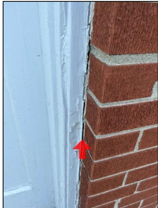
Caulking - deteriorated, loose or missing
