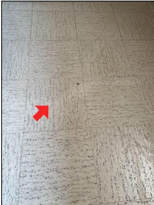
Possible asbestos containing materials
