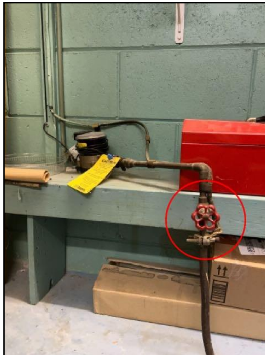
Water shut-off valve
