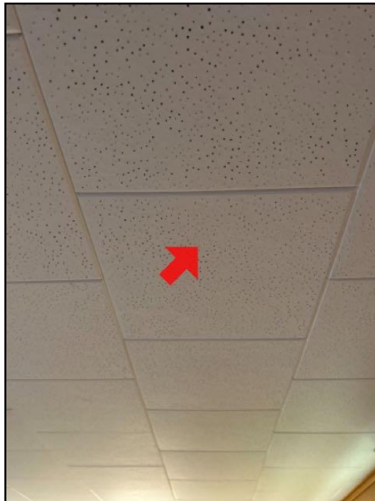
Possible asbestos containing materials
