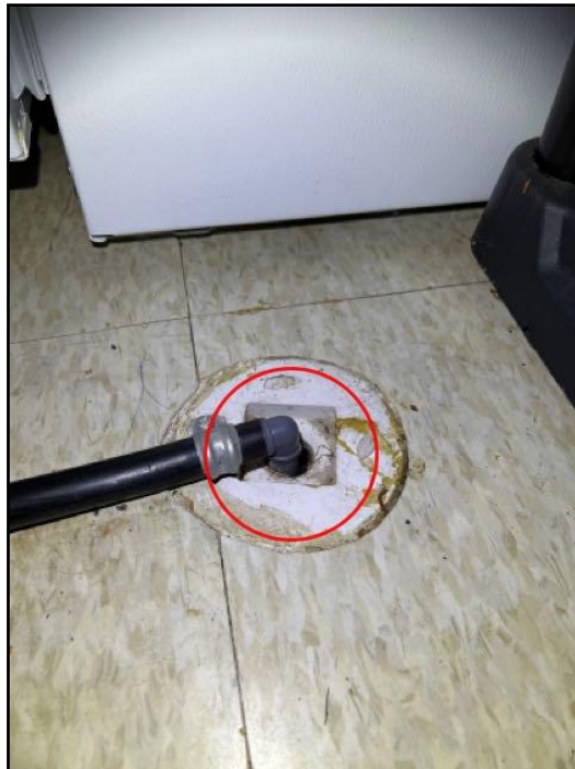
Condensate drains into clean-out
