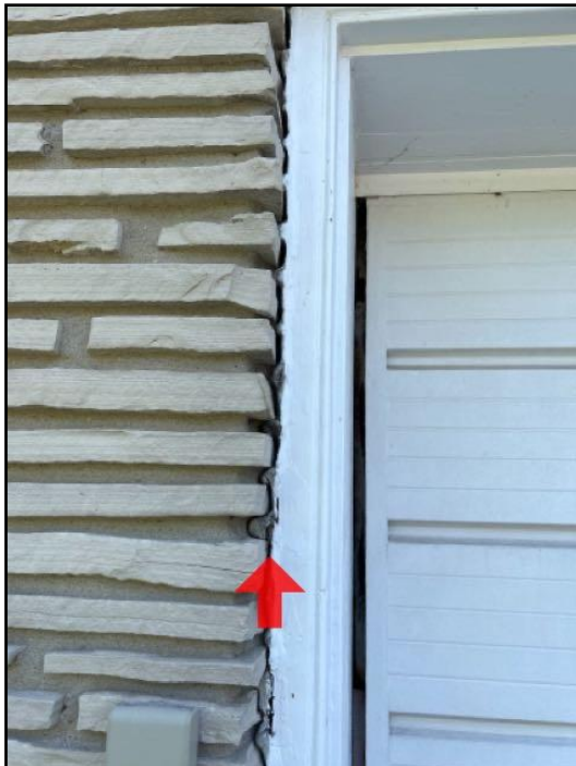
Caulking - deteriorated, loose or missing
