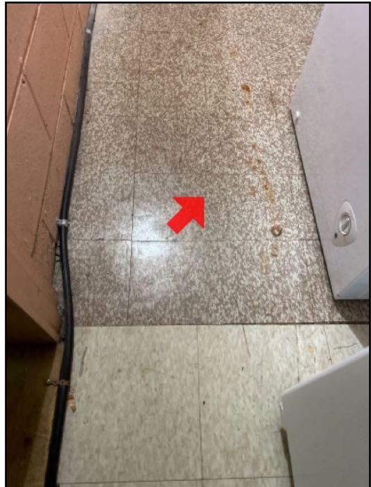
Possible asbestos containing materials
