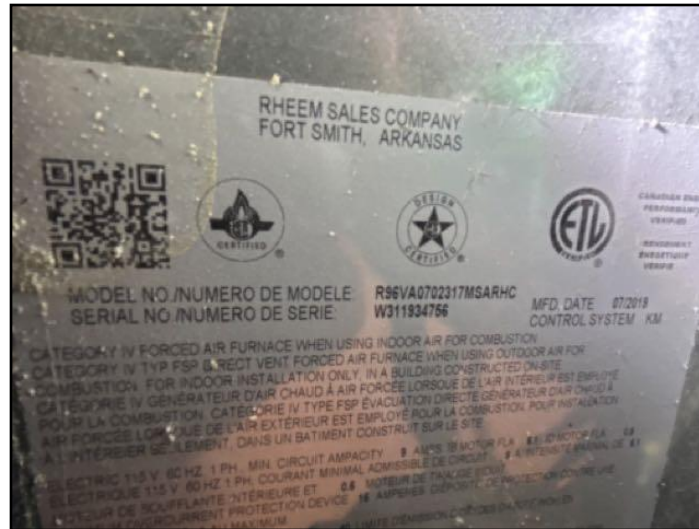
Furnace data plate
