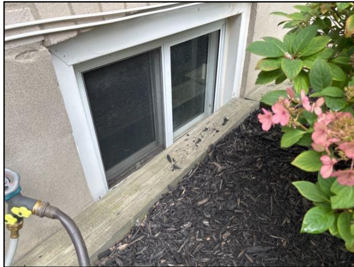
Window well needed
