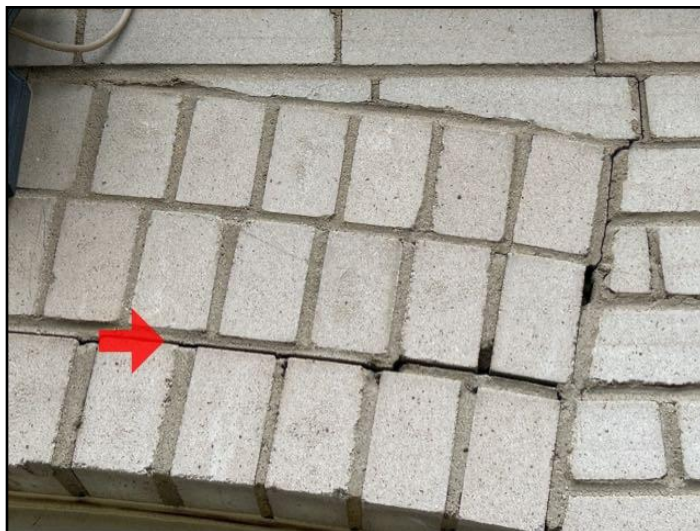
Typical minor cracks
