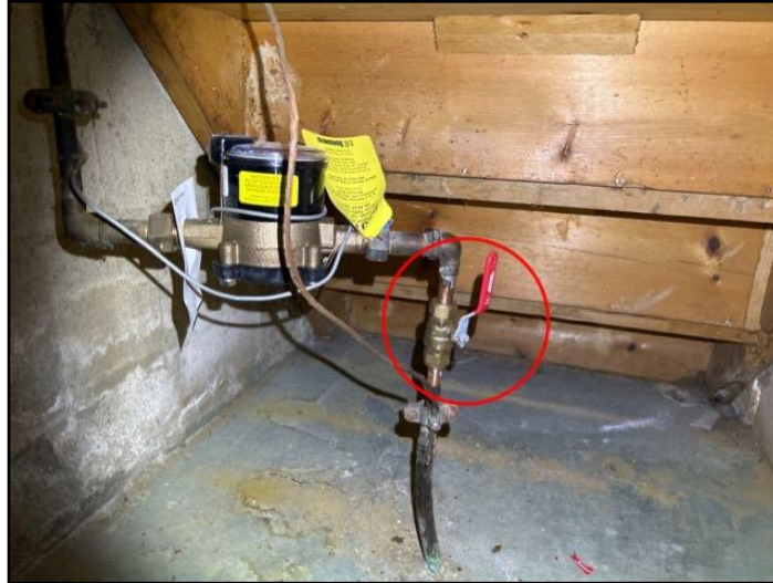
Water shut-off valve
