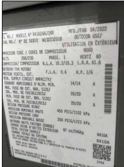
Air conditioner data plate
