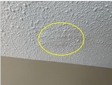
Living Room ceiling below bathroom
