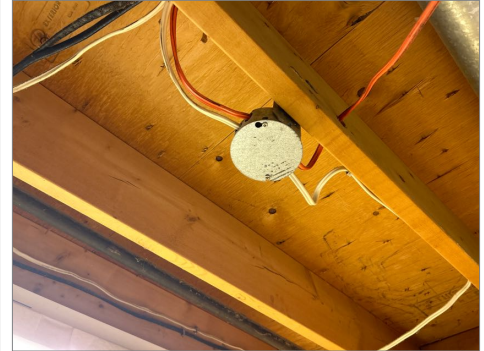
Basement Utility room
