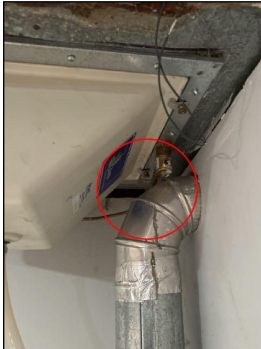
Access blocked by duct
