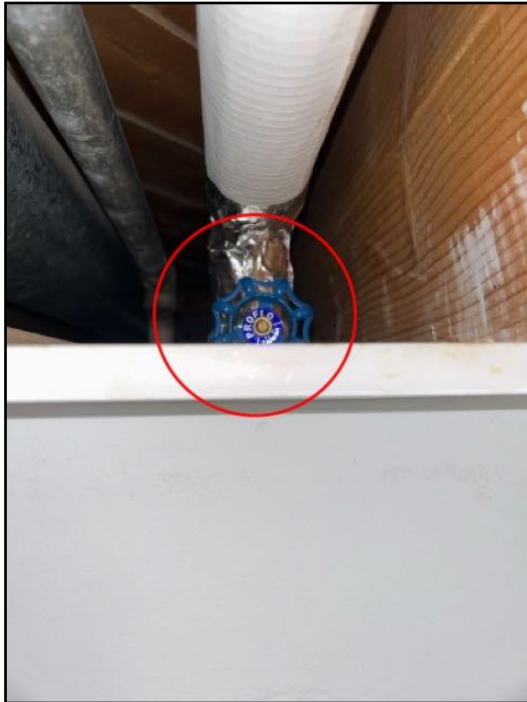
Water shut-off valve
