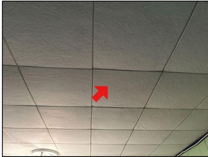
Possible asbestos containing materials
