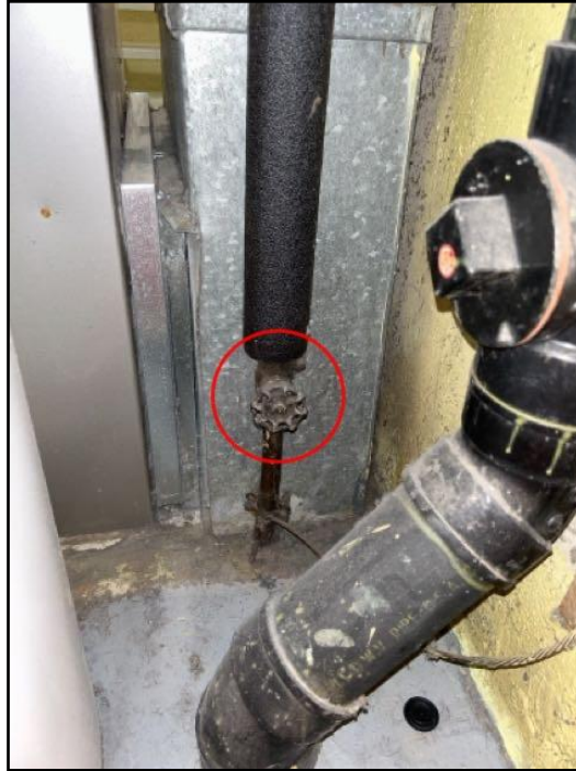
Water shut-off valve
